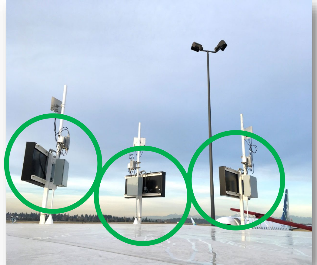
Ramp / PLB Wi-Fi Access Points
